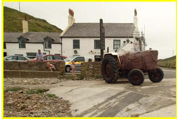
Low wall at edge of pub car park in fair condition (Asset Ref No. 1221C901C0704C05)
