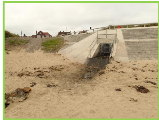
Partly blocked outfall at south east end of seawall Asset ref No. 1221C901C0603C01
