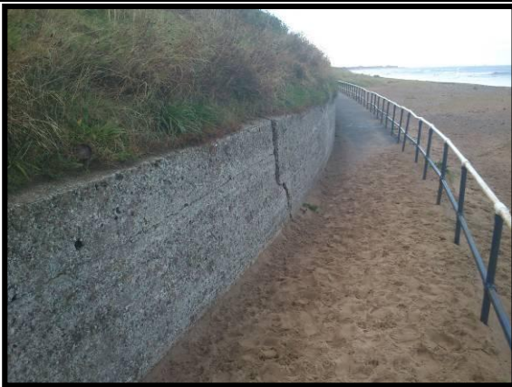
Crack in concrete wall below coastal slope (Asset Ref No 12221C901C0702C03) Photo from 2010 report.
