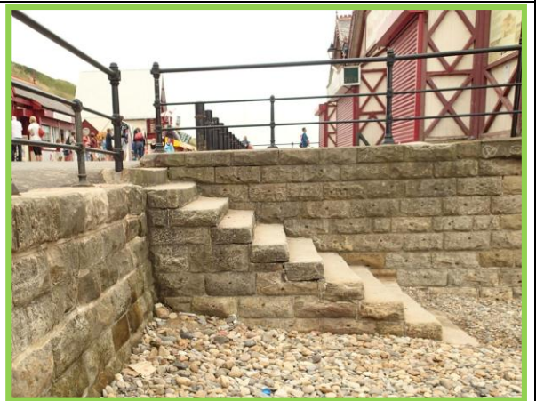
Loss of filler below steps requires re-pointing (Asset Ref No 1221C901C0704C04)
