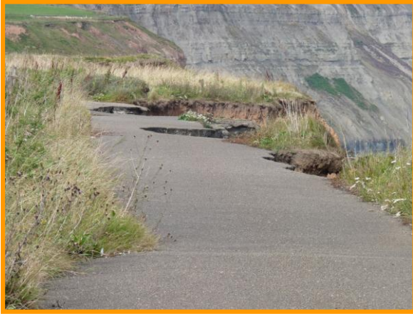
E59/3 ongoing recession of cliff top through old road (Partly Active)
