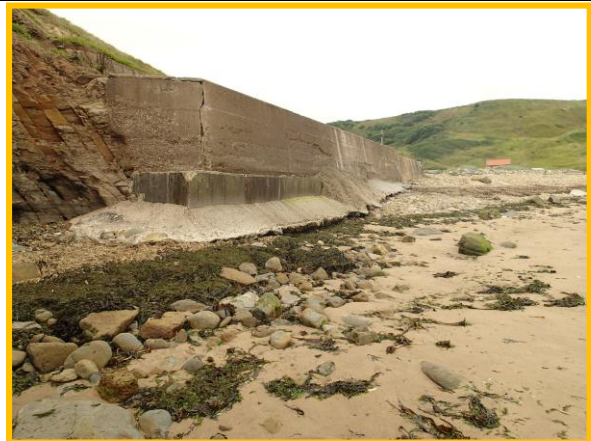
Undermining of wall toe exposing deep voids. (Asset Ref No. 1221D901D0202C03)
