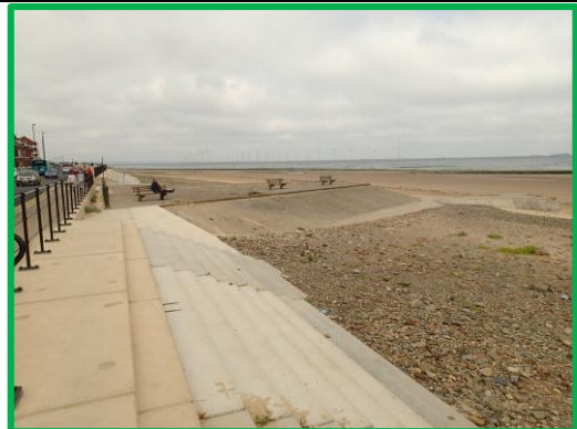
View of eastern end of main Redcar Seawall. Asset ref No. 1221C901C0602C01
