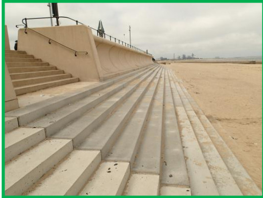
New stepped revetment and wave wall at west end of Redcar, Asset ref. 1221C901C0602C06
