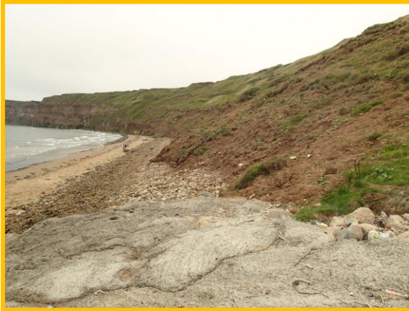
Poured concrete repairs at east end of defence adjacent to slumping cliffs (Asset Ref No. 1221C901C0704C05)
