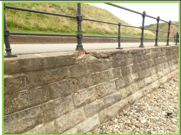
Damaged section of coping towards western end of wall (Asset Ref No 1221C901C0704C04)
