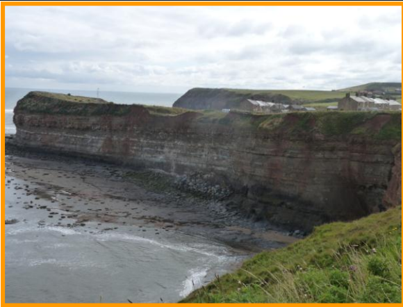
E60/1b ongoing rockfall from lower cliff and localised failures of overlying till (Partly Active)
