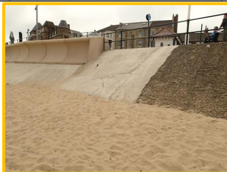
Interface with new seawall at the eastern end of Asset Ref No 12221C901C0601C01
