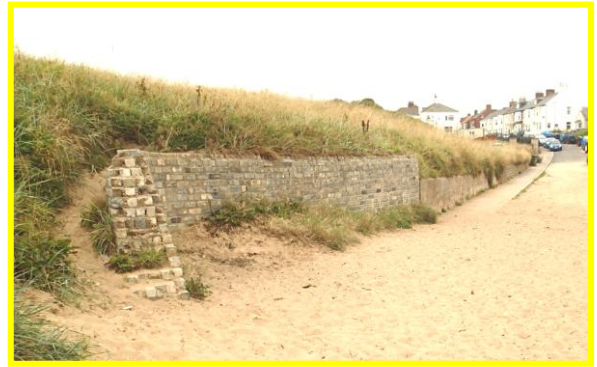
Missing masonry at seaward end of wall to southeast of beach access. (Asset Ref No 12221C901C0702C01)
