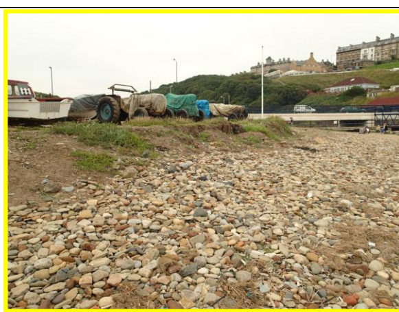
Erosion of cobble bank adjacent to boat park. Asset Ref No 1221C901C0704C02
