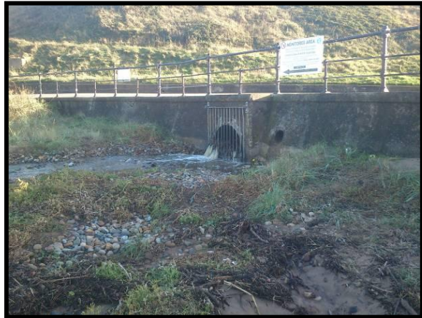
Partially blocked outfall exiting through sea wall at Hazel Grove Photo from 2012 report (Asset Ref No 1221C901C0703C02)
