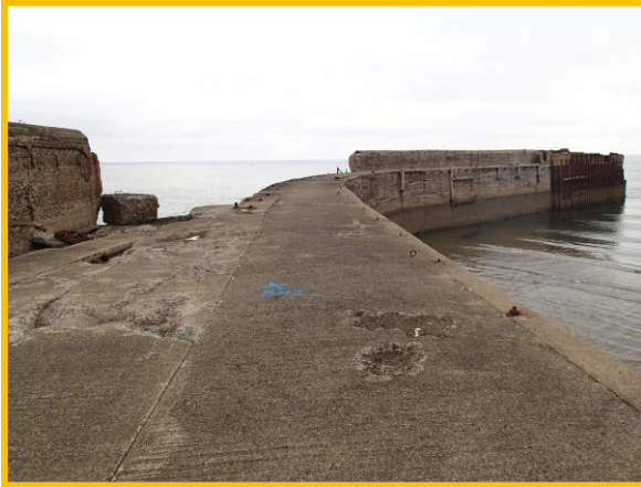
View of crest from access gate showing missing section of crest wall. (Asset Ref No. 1221D901D0201C02)
