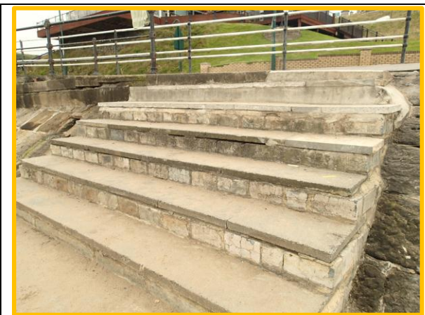
Repaired steps to beach have cracks beneath treads (Asset Ref No 1221C901C0704C01)
