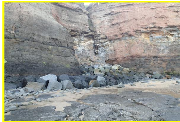
Western section of rock armour at cliff toe next to Cowbar lane Photo taken 12/09/2014 (Asset Ref No. 1221D901D0401C01)
