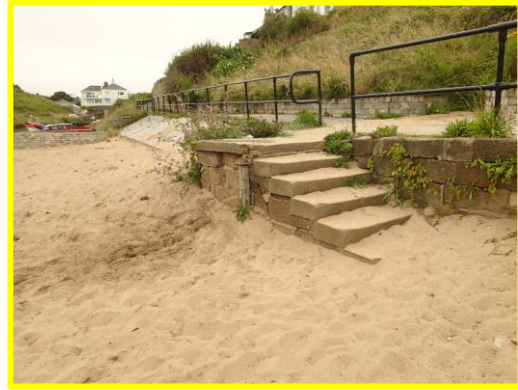
Missing mortar in joints and vegetation growth. (Asset Ref No 12221C901C0702C03)
