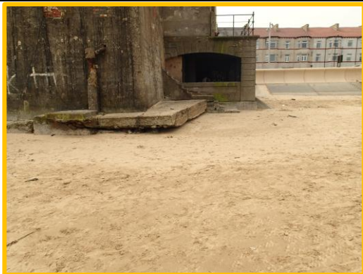
Undermining of toe apron at cinema seawall Asset ref No. 1221C901C0602C05
