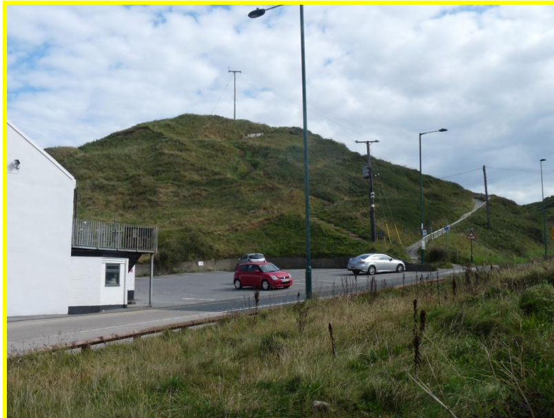
E53/5 slumped in 2012, leaving open cracks in the cliff face which are still visible. Locally Active. Photo August 2014
