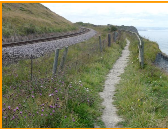
E54/3a proximity of footpath and railway line to actively eroding cliff top (Partly Active) Photo August 2014
