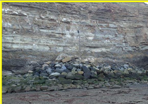
Eastern section of rock armour at cliff toe next to Cowbar lane Photo taken 12/09/2014 (Asset Ref No. 1221D901D0401C01)
