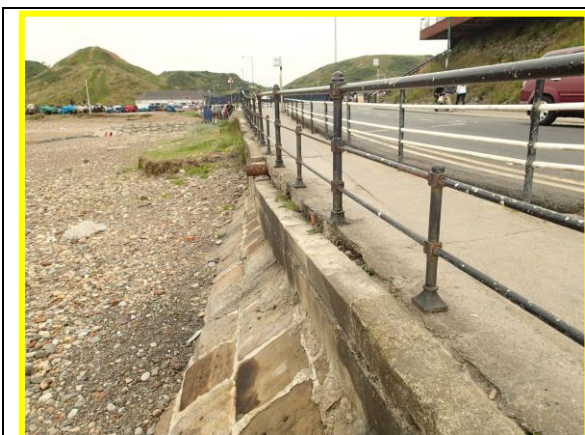
Damage to coping stones to edge of path by road. (Asset Ref No 1221C901C0704C06)
