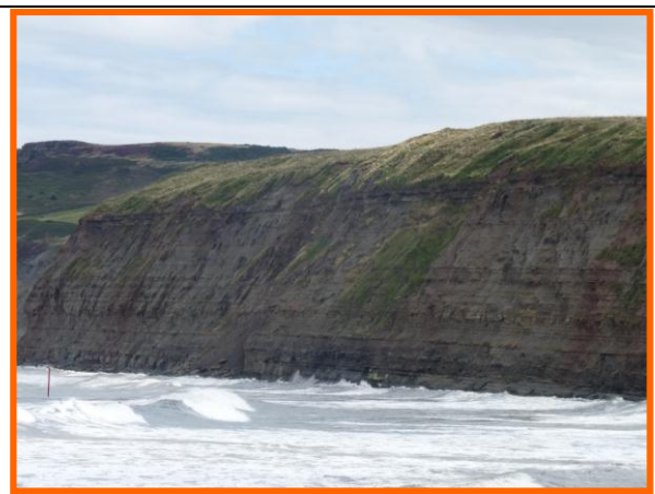
E57/6 This unit has been upgraded because the majority of the lower and mid-cliff is active and there is evidence of failure from upper cliff. (Partly Active)
