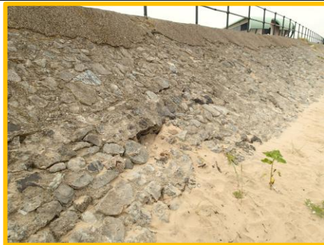
Damaged area of revetment (Asset Ref No 12221C901C0601C01)
