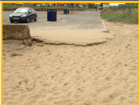
Damage at access ramp adjacent to west extent (Asset Ref No 12221C901C0601C01)
