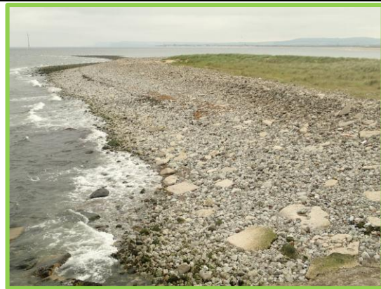
Slag bank running south east from South Gare with debris from failed sections of breakwater (Asset Ref No 12221C901C0506C01)
