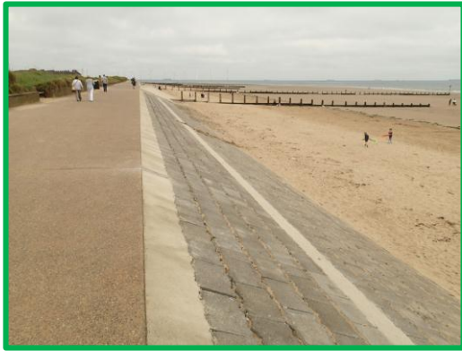
Concrete block revetment and concrete promenade in very good condition. Asset ref No. 1221C901C0603C01
