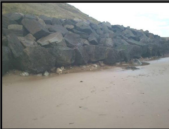
Photo from 2012 report showing low beach levels have exposing toe of rock armour to scour damage (Asset Ref No. 1221D901D0202C01)
