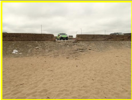
Gap in concrete wall and exposed revetment (Asset Ref No 12221C901C0601C01)
