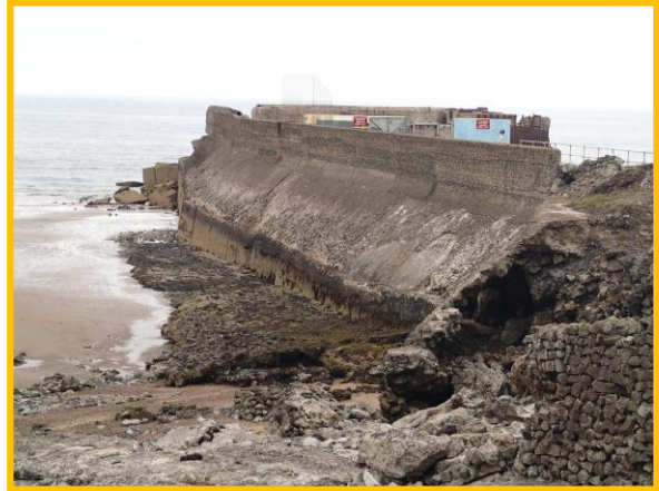
Voiding and collapse of west side of jetty structure (Asset Ref No. 1221D901D0201C02)
