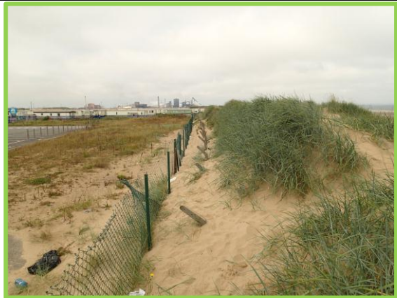
E52/11 Further accretion and roll back of dunes next to former site compound at Coatham
