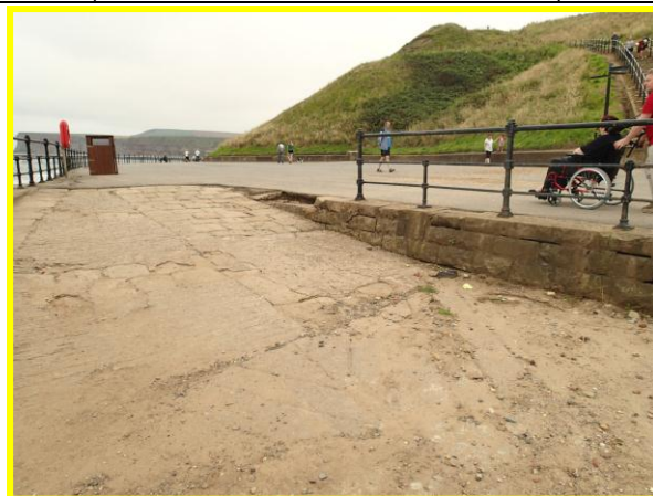
Missing coping stones at edge of ramp at Hazel Grove Foot (Asset Ref No 1221C901C0703C02)
