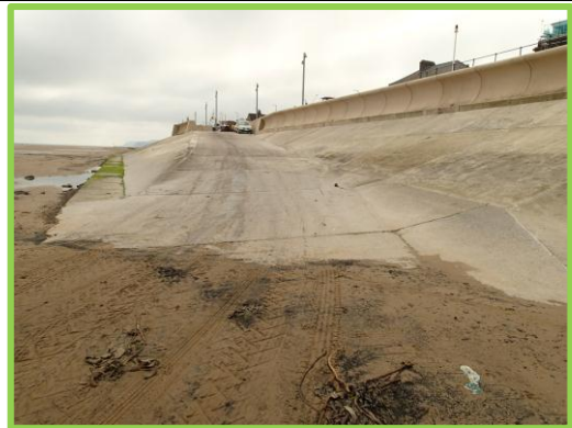
Low beach levels adjacent to boat park slipway Asset ref No. 1221C901C0602C02
