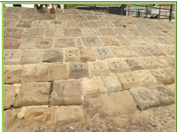
View of sloping masonry revetment at car park area. (Asset Ref No 1221C901C0704C01)
