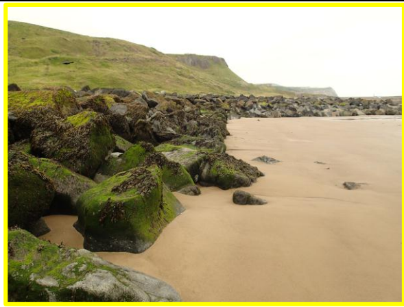
Area of displaced and loosely packed armour on seaward side of fishtail (Asset Ref No. 1221D901D0202C05)
