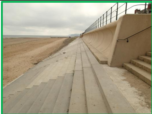
Stepped seawall and wave wall in very good condition. Asset ref No. 1221C901C0602C01
