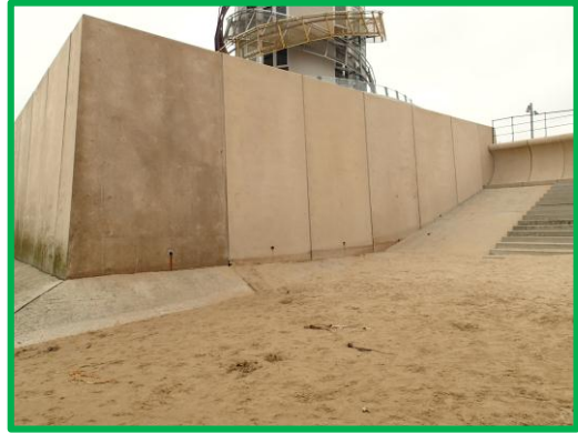
New vertical wall at the Beacon tower reconstructed in 2012, Asset ref No. 1221C901C0602C03
