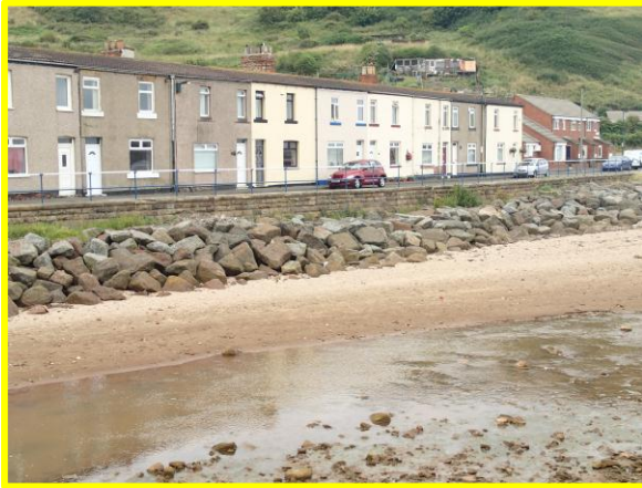
Rock armour and low sea wall in front of properties (Asset Ref No. 1221D901D0202C02)
