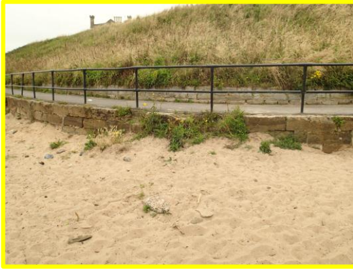
Missing coping blocks and open joints in masonry blockwork in wall below path. (No change from 2012) (Asset Ref No 12221C901C0702C03)
