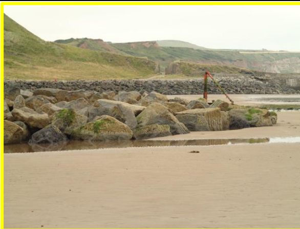
Seaward end of fishtail breakwater showing damaged navigation marker (Asset Ref No. 1221D901D0202C05)
