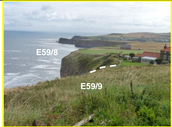
E59/9 (Locally Active) and E59/8 (Partly Active) – Limited activity at the cliff top in front of the cottages at Boulby which increases south-eastwards.
