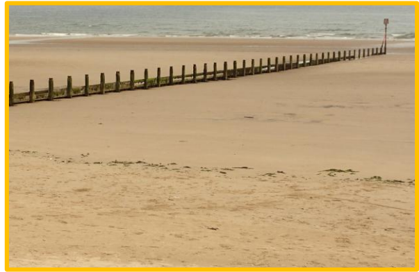
Many groynes refurbished in 2012 have missing planks. Asset ref No. 1221C901C0603C01
