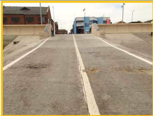
Localised damage to slipway at the RNLI building Asset ref No. 1221C901C0602C02
