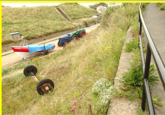
Extensive vegetation growth on revetment; (Asset Ref No 12221C901C0702C02)
