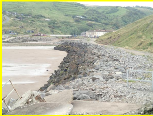
General view of revetment looking from Jetty towards village (Asset Ref No. 1221D901D0202C01)
