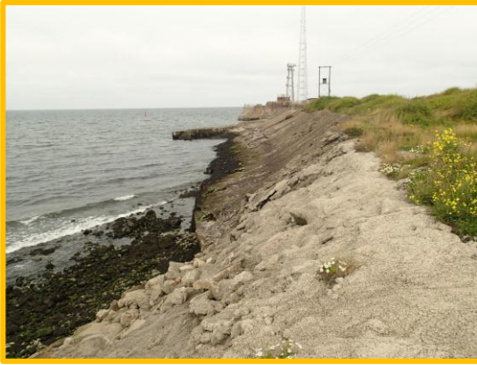
Patchwork of repairs on west side of South Gare Breakwater, (Asset Ref No 12221C901C0506C01)
