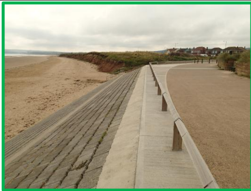
View towards eroding cliff at east end of seawall Asset ref No. 1221C901C0603C01, (with 1221C901C0701C01 in distance)
