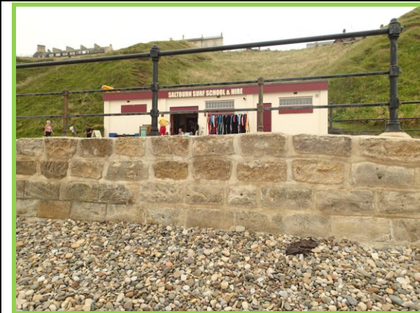
Example of area where blockwork has been recently repaired (Asset Ref No 1221C901C0704C04)
