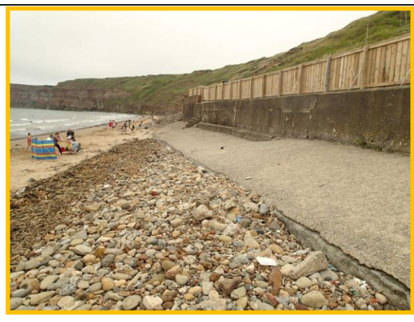
Higher beach levels at time of 2014 inspection affording some protection to defence. (Asset Ref No. 1221C901C0704C05)
