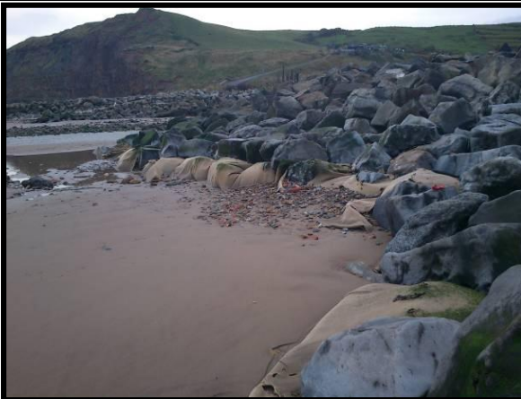
Photo from 2012: Exposed geotextile matting at rock armour toe. (Asset Ref No. 1221D901D0202C02)
