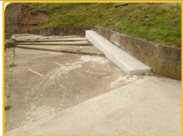
Wall crest showing repairs and eroding cliff to east in background. (Asset Ref. No 1221D901D0202C03)
