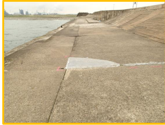
Patchwork of repairs on east side of South Gare Breakwater, appear to be holding but facing to outer structure missing (Asset Ref No 12221C901C0506C01)
