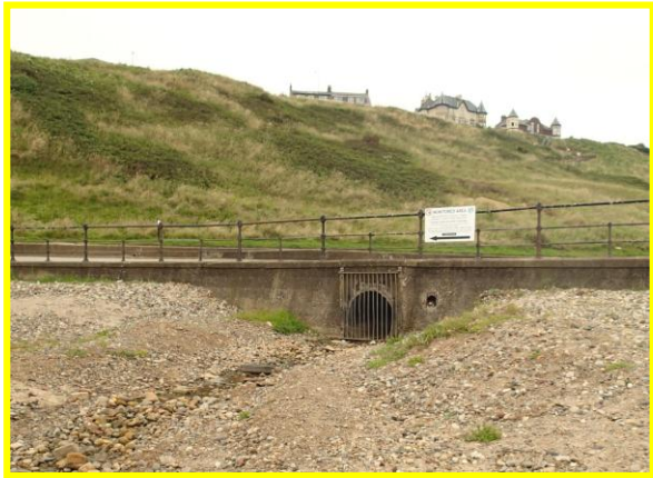
Outfall exiting through sea wall at Hazel Grove sea wall at Hazel Grove Foot 24 July 2014 (Asset Ref No 1221C901C0703C02)
