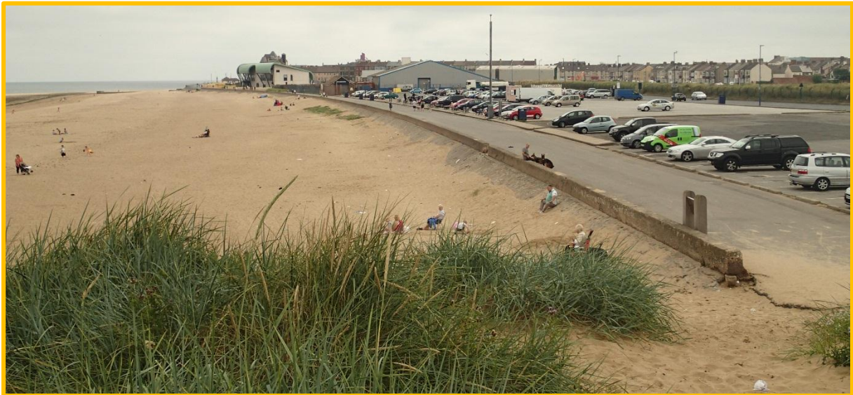
Overview of defences at west of Redcar from east end of sand dunes. (Asset Ref No 12221C901C0601C01)
