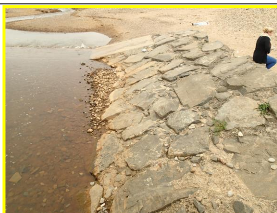
Lower beach levels to east side of beck had exposed the crest of the rock armouring (Asset Ref No 1221C901C0704C06)
