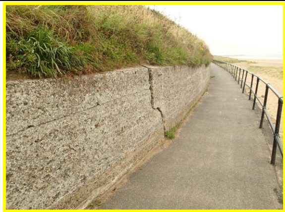
Crack in wall no change from 2010– photo from 24/07/2014. Note lower beach levels. (Asset Ref No 12221C901C0702C03)
